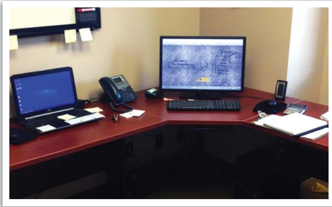
WWTP SCADA system runs on a desktop at the City of Tehachapi admin office.
