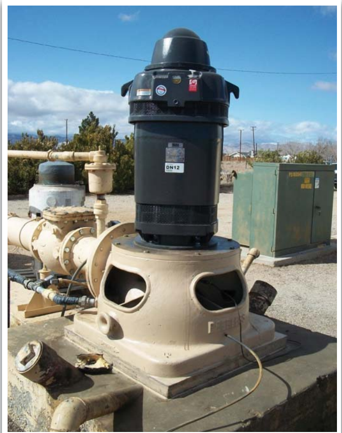
Retrofitted Water Well Pump 15A
